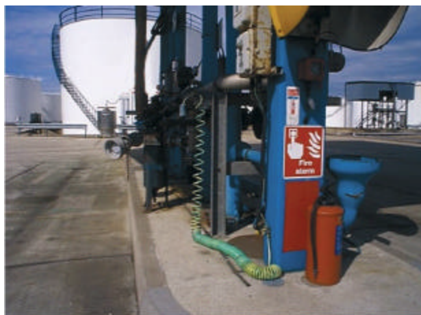
Typical truck loading area with grounding connection, fire extinguisher, and fire alarm switch
